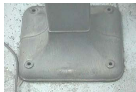
Picture shows machine not anchored to floor Image courtesy of OSHA
